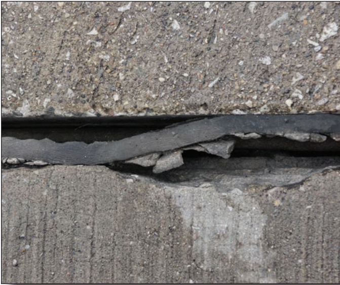
Figure 2. In cold weather, joints open to allow intrusion of incompressible materials
