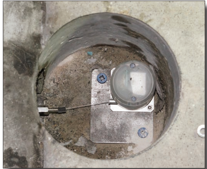
Figure 3. String-pot sensor has integrated data-logger to monitor long-term displacements
